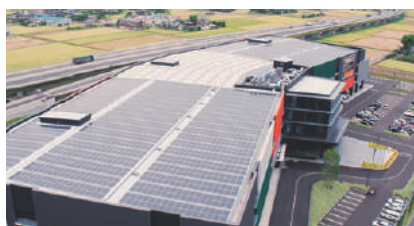
Solar panels installed on the roof of Planet Saitama
